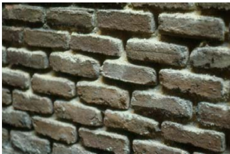
fig. 3 descarnado (scraped wall)
