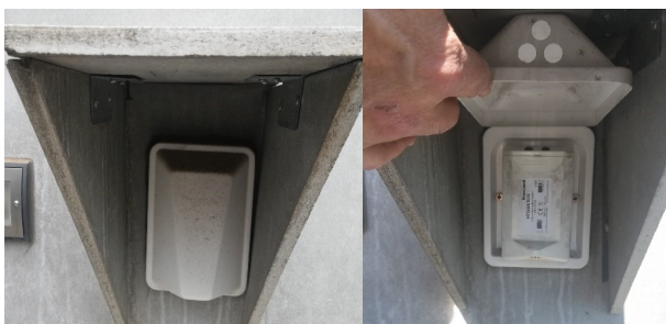
Figure 5: Honeywell - H7508A1042 - Outside Air Humidity Sensor. Apolonio Morales 29, Madrid, Control System. Source: Self-elaboration.
