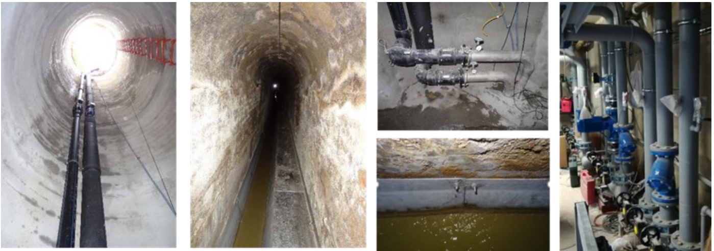
Figure 15b: Connection installation between the Interchanger integrated in the municipal collector and the technical room of the indoor pool. Source: Eneres.
