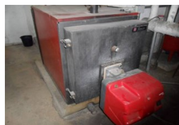
Pool water heating
