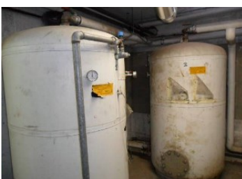
Hot water Production
