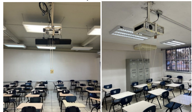
Fig. 5. Installation of HOBOT Data Logger sensors in classrooms of buildings. Own photos, 2023.
