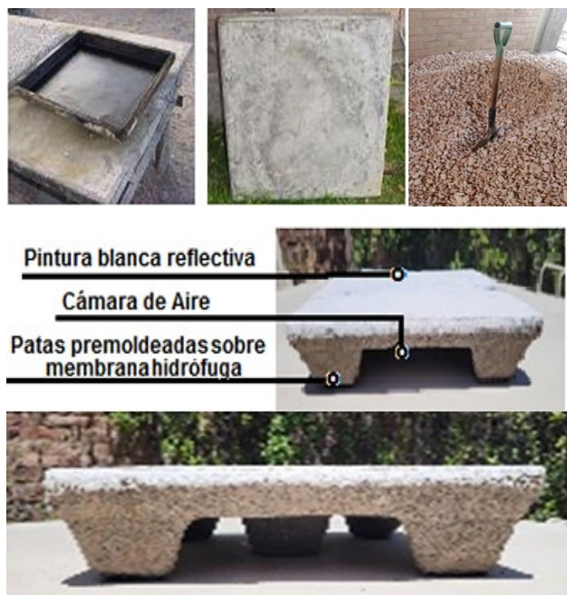
Fig. 11. Views of the pomeca, mold on vibrating table and plate of the precast ceiling mounted on the roof.
