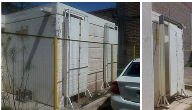
Fig. 14. Views of the Laboratory next to the prefabricated thermo-insulating envelope system integrated in the sensor installation stage.
