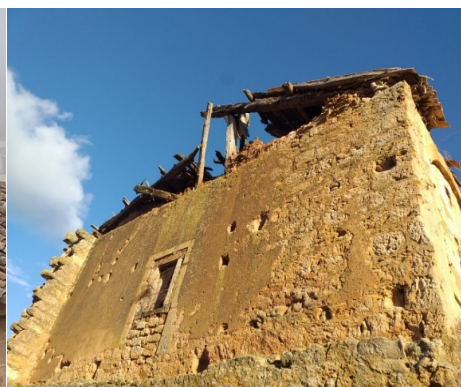
Fig. 7. Damage to the facades due to the collapse of the roofs (Source: Paula Montoya Saiz)
