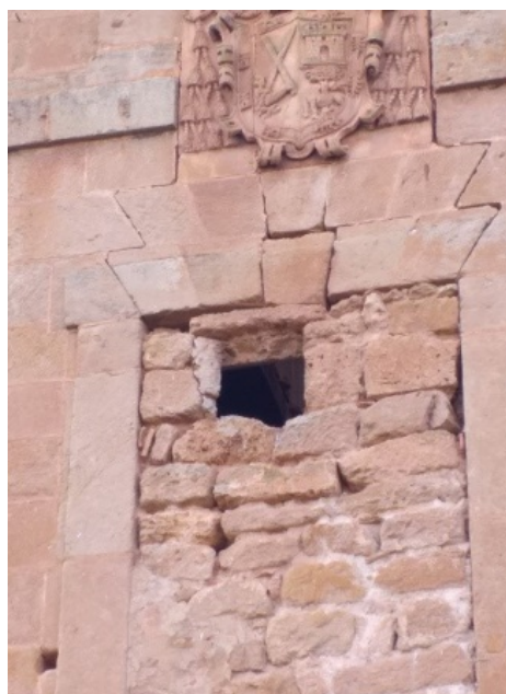
Fig. 8. Cracked lintel and blinded gap. (Source: Paula Montoya Saiz)
