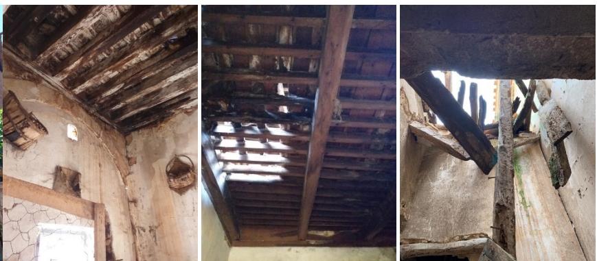
Fig. 5. Generalized deterioration of the slabs. (Source: Paula Montoya Saiz)
