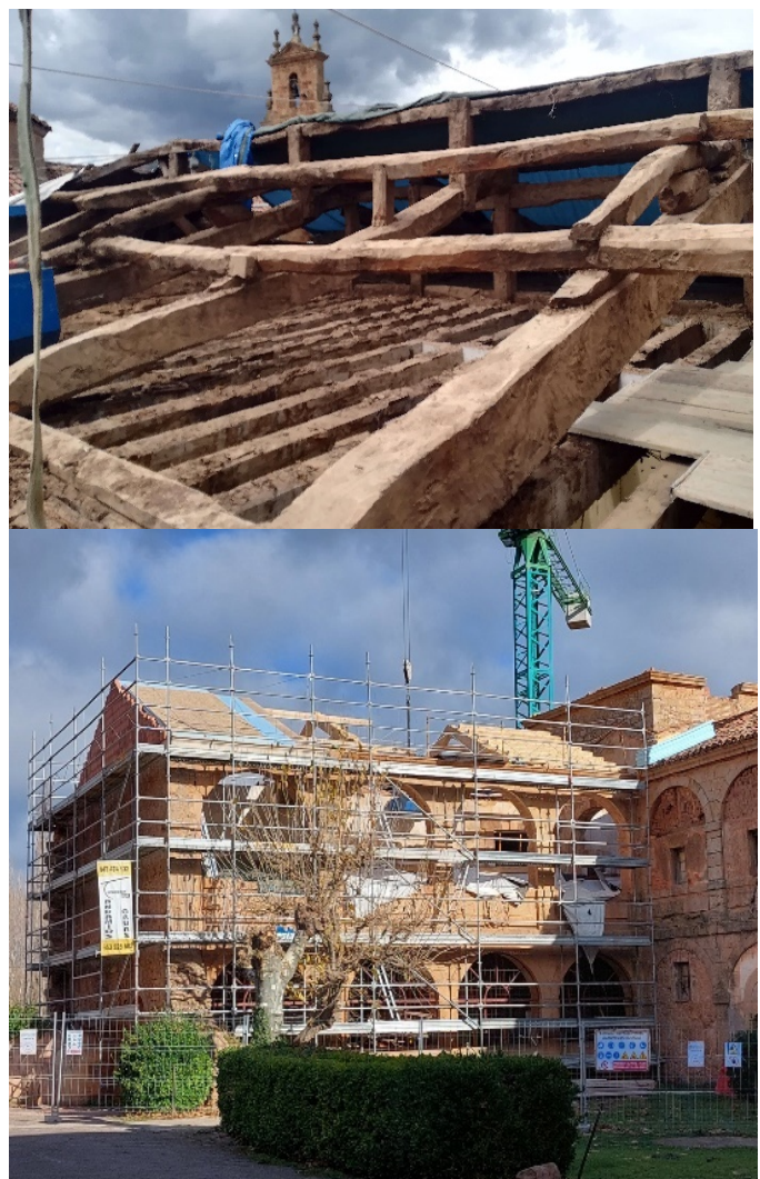
Fig. 13: Dismantling of the old roof and assembly works of the new one. (Source: Paula Montoya Saiz)
