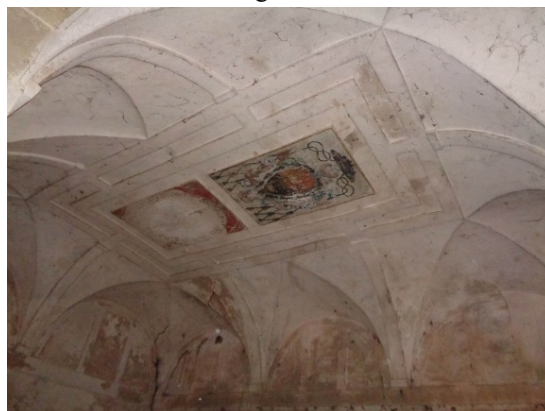
Fig. 2. Partitioned vaults over the main staircase. (Source: Imanol Ruiz de Vergara Ruiz de Azúa)
