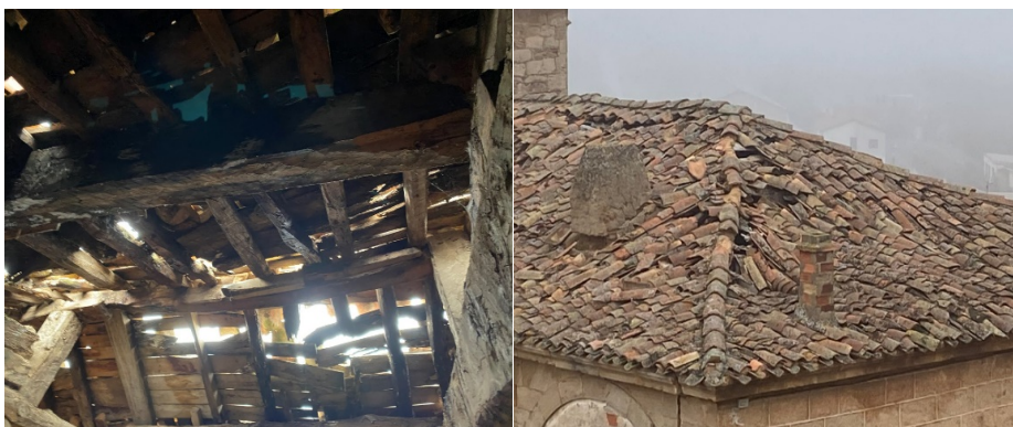
Fig. 6. Damage to the roofs. (Source: Paula Montoya Saiz)
