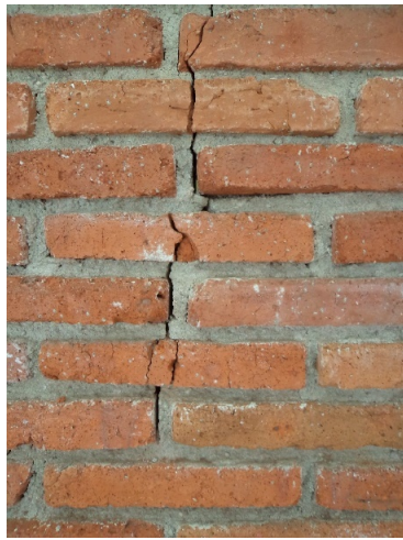
Fig. 4. Crack in facing brick façade. Source: https://www.redpiso.es/news/los-vicios-ruinogenos/
