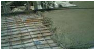
Fig 8: Implementation of concrete slab on Ro fix and beams in flat roof (source:17)
