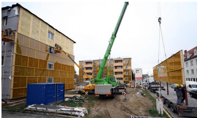
Fig. 1. Installation of large panels on Dieselweg building, Graz (Austria). The installation takes place by means of truck-mounted cranes and mobile cranes.
